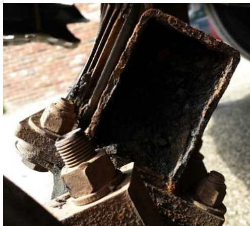
Figure 2. Rusted Swing Frame Cross Beam
